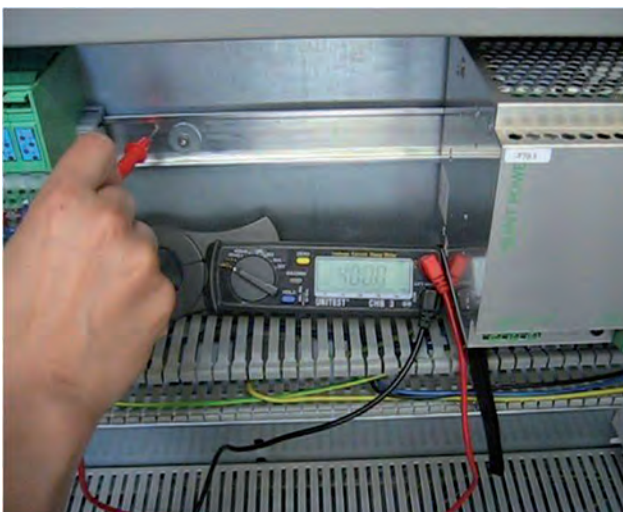
Figure 4: Detection of earthing contact problems caused by oxidation processes using a clip-on ammeter (Photo: IVG Göhringer)
