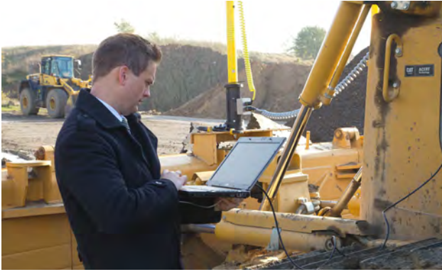
Figure 3: Dennis Blume from ifm on site: The controller was tested on the machine and the programming adjusted again and again (Photo: ifm)
